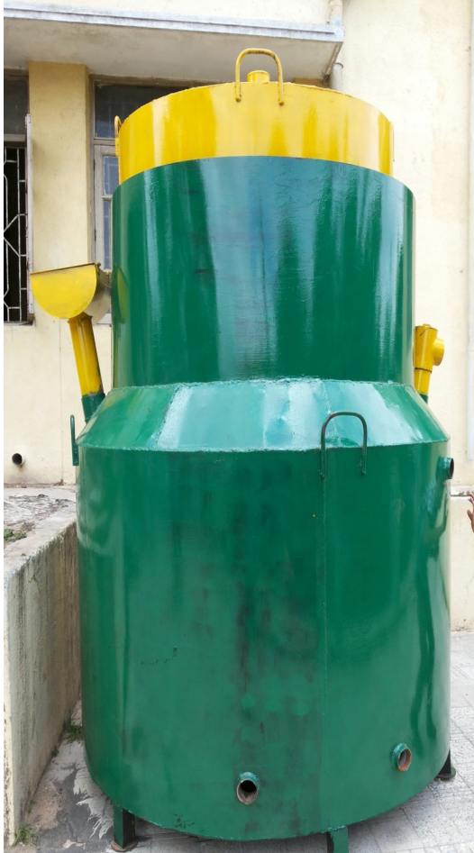
Prefabricated- Mild Steel Kitchen Waste Biogas plant of capacity 50kg per day at Sri Chamundeshwari Temple, Chamundi Hills, Mysore
