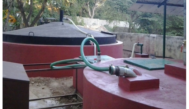
1500 kg.day input biogas plant at Mysuru Zoo.
